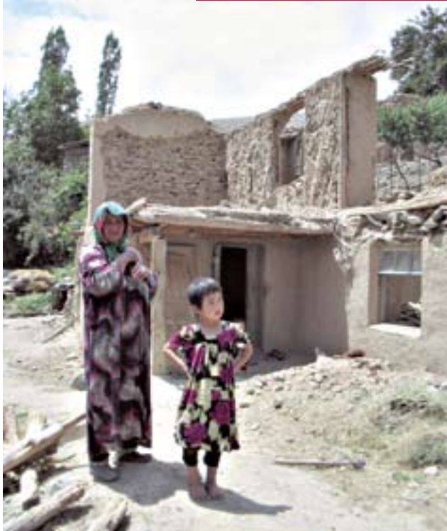
Saidbibi and the rest of her family watched as their house collapsed and their possessions were carried away by the mud.
